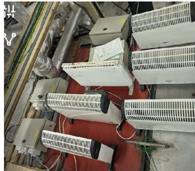
Bank of heaters ~12kW
