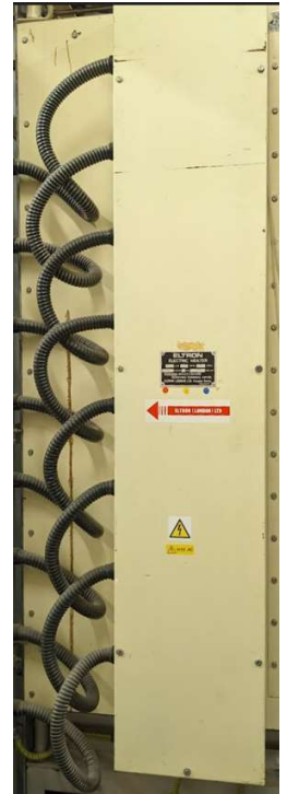
Inlet Heaters 405kW
